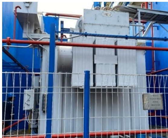
Figure 1. Unit Station Service Transformer
