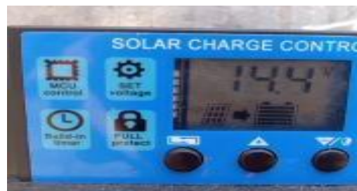
Gambar 3. Proses pengecekan Solar Charger Controller (SCC)
