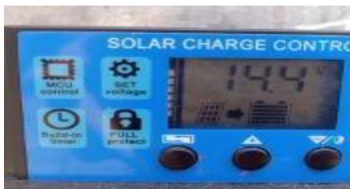
Gambar 3. Proses pengecekan Solar Charger Controller (SCC)
